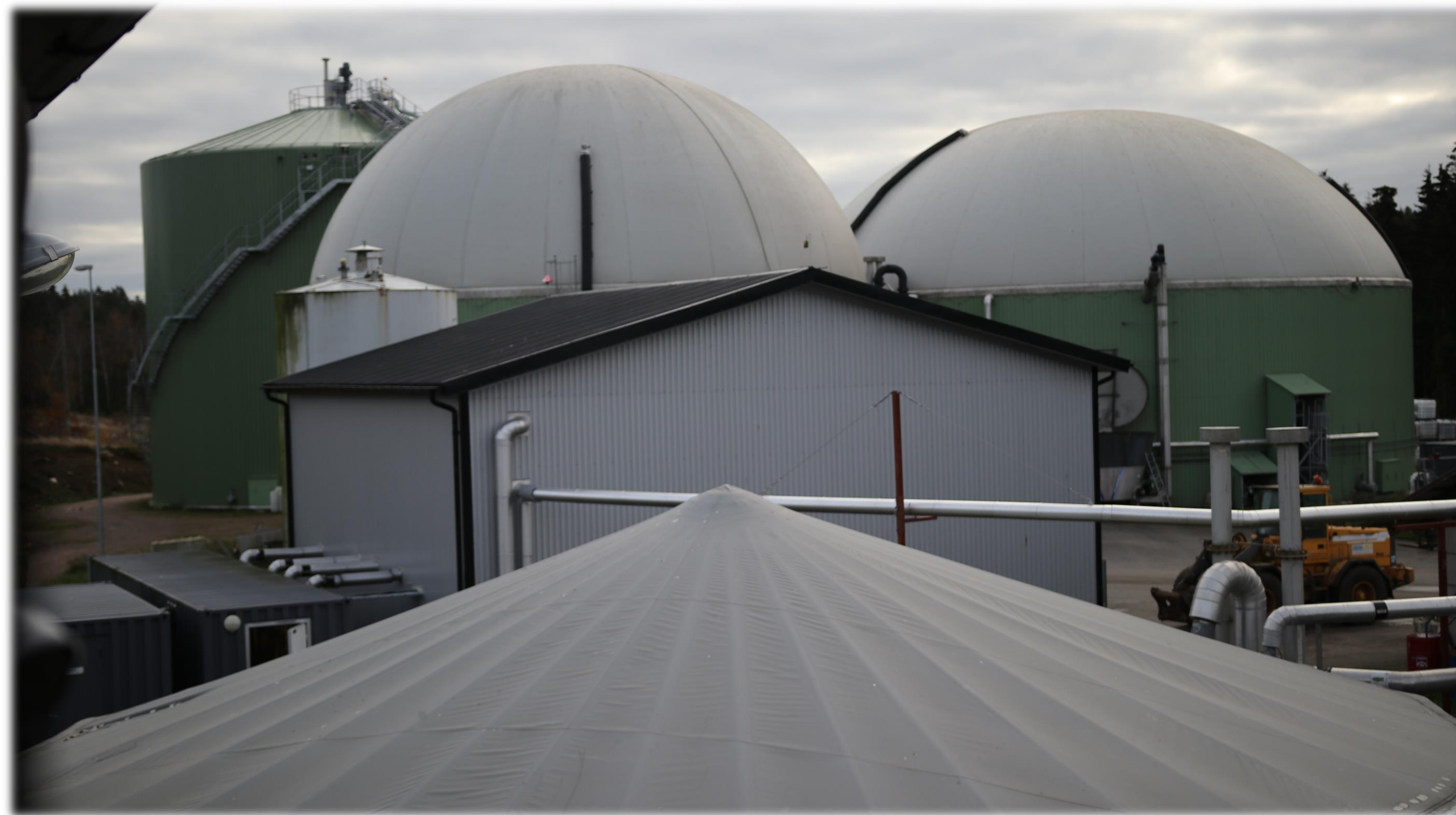
Overview of biogas plant in Vårgårda-Herrljunga Biogas AB in Vårgårda, Sweden
